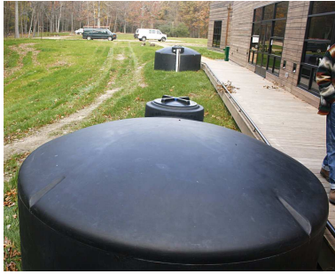
Right: Cisterns used to collect water from the roof of the center.
